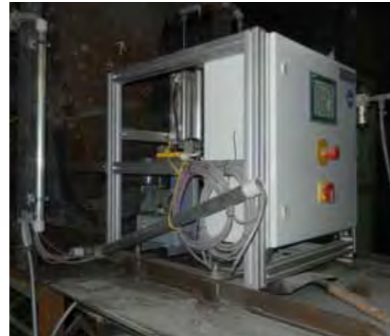
SPC in a steel foundry
